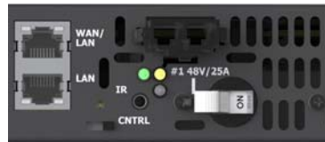
Power level is good, but approaching limit
