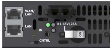
Power level is good and can add more panels.
